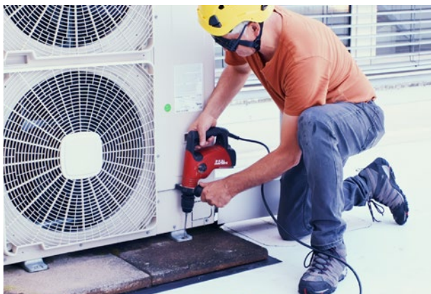
Drilling holes into roof waterproofing membrane by installing various equipment after completed application.
