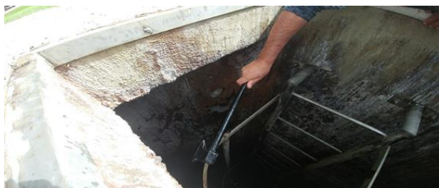
Fig. 9: Picture taken in Israel where a system similar to Scenario-2 has shown premature failure after just 5 years in service.
