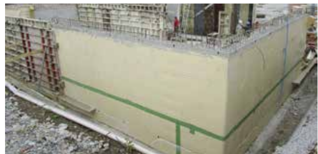
Open excavation with SikaProof® A, after removing the formwork the anchor penetrations has to be sealed.
